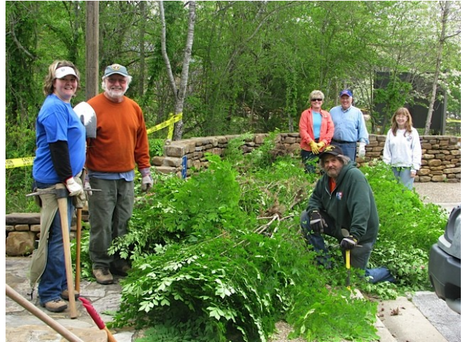
Large bushes surrounding the Tyler Bend Visitor Center ready to be hauled away by volunteers. Picture by Jack Stewart
